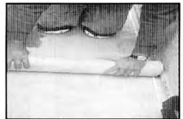
4 Place GOLD into bonding material. Allow 2" overlap to all adjacent sheets and flashings
