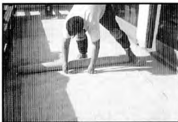
2 Pre-cut GOLD to fit layout. For waterproofing, pre-cut flashing pieces save time in tight space
