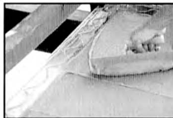
3 Use Latex Thin Set for bonding, mix per manufacturer's instructions. Set tile after full mortar cure
